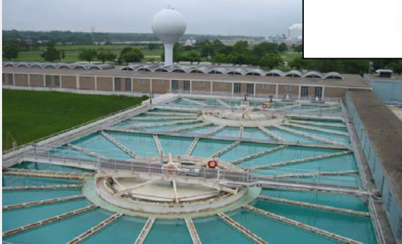
Miami Water Treatment Plant
